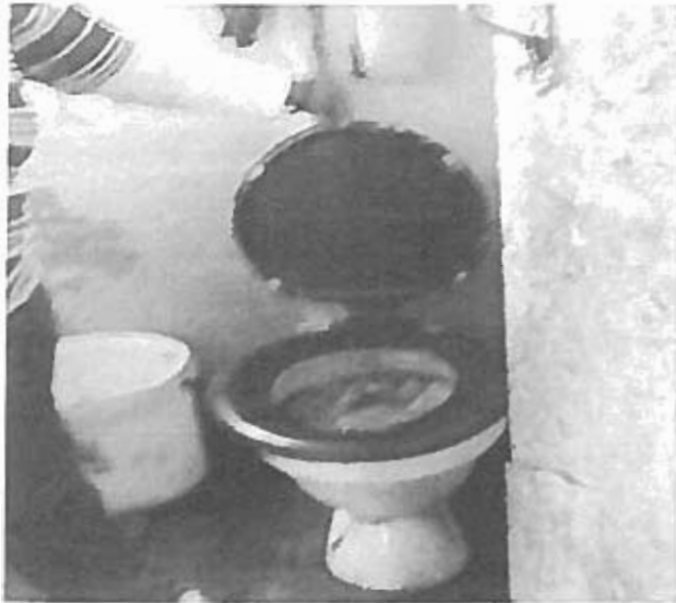
Photograph 2 shows a blocked toilet resulting from the outdated waste water disposal system.
