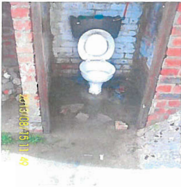
Photograph 1 showing a broken and inaccessible toilet surrounded by water following heavy winter rains.
