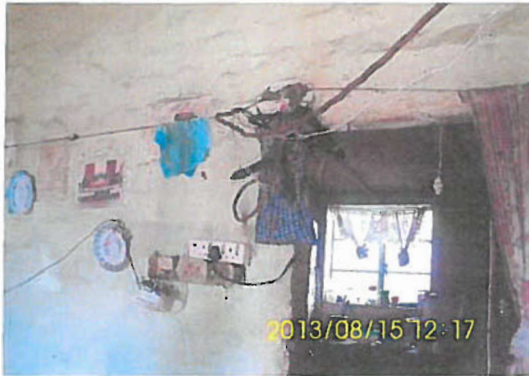
Photograph 4 depicts unsafe electrical switches and sockets which were a common feature.
