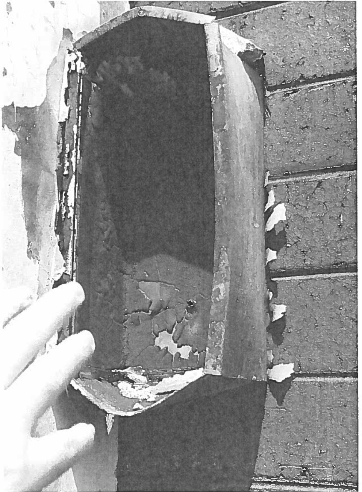
Photograph 7: The empty wall mount for the gas hooter
